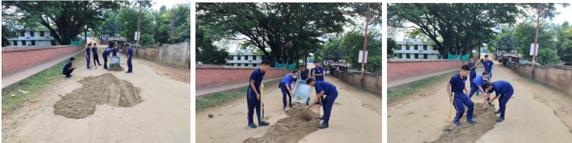
27 th September 2022, NCC (SD) Boys organised Social work and repaired the College approach road
