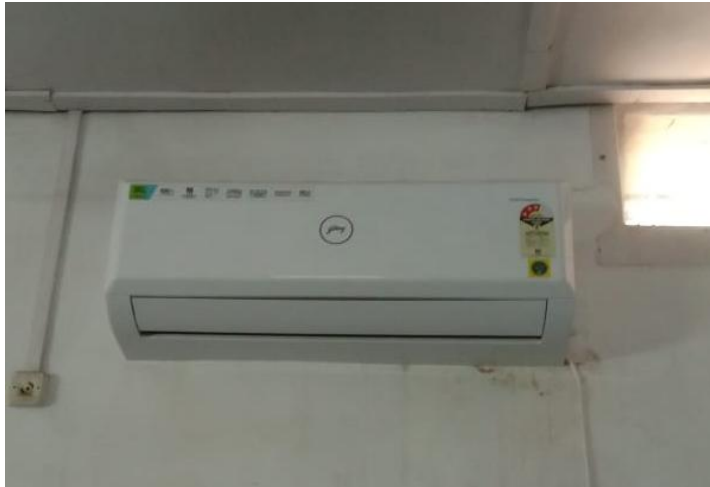
Photograph 7: AC Unit for Vice Principal's Office (One Unit; 2 Ton)
