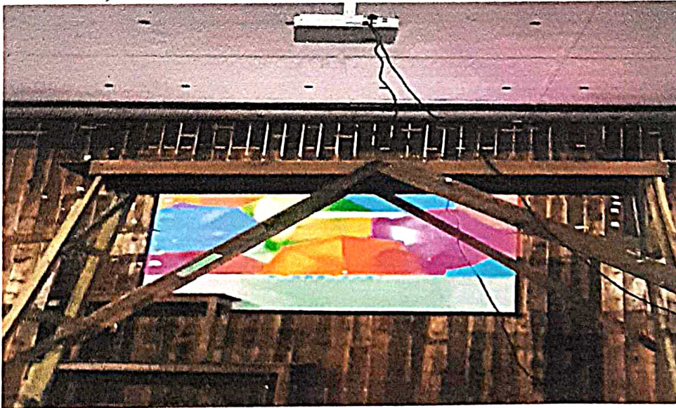
(Projector installed in Auditorium)
