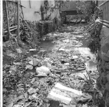
Area is covered with solid waste
