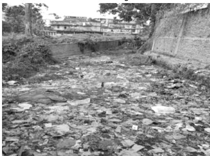
Drain covered by solid waste and sediments
