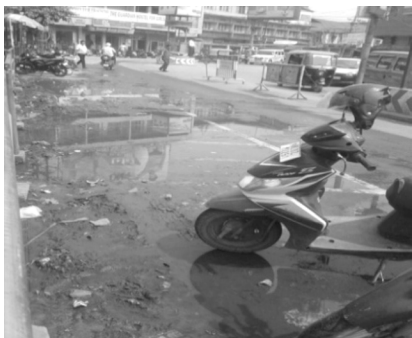
Over flow of water from the drainage due to blockage
